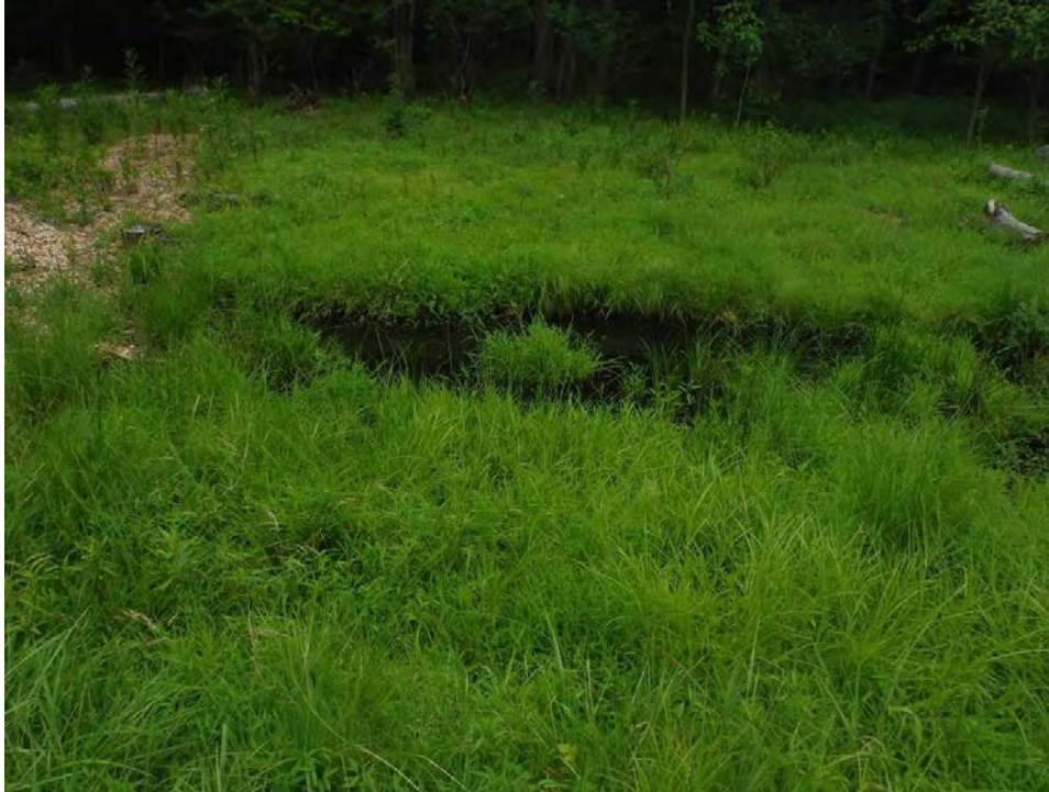
Figure 10: Standing Water at the Toe of the Polishing Pond's South Embankment
