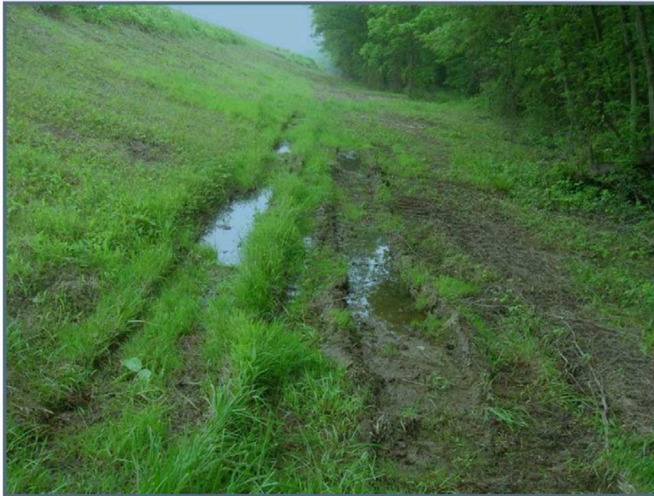
Photo 1 – Wet area at toe of the East Embankment, looking north from Sta 0+30. (2009 annual inspection)
