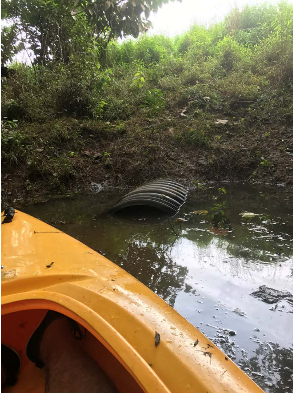
Figure 13: Unauthorized Discharge Pipe near Black Gut Creek
